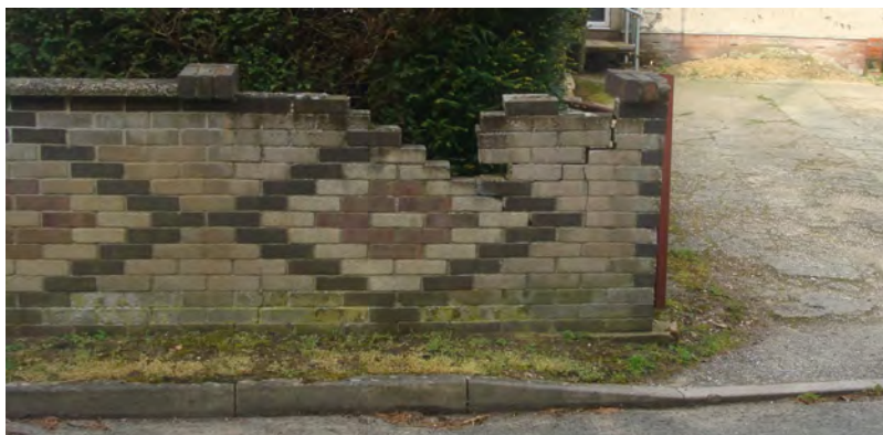
Picture 1.18 Modern decorative wall in very poor condition
