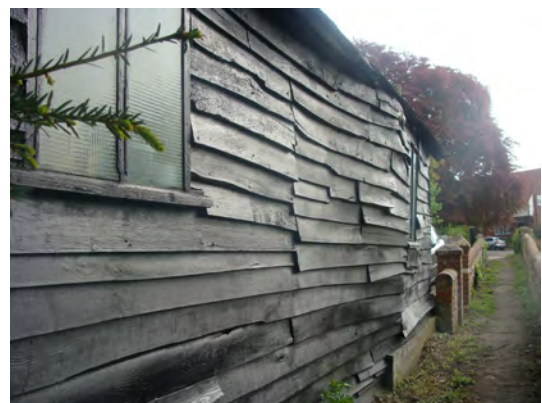
Picture 1.14 Weatherboarded barn of historic value within curtilage of the Old Vicarage
